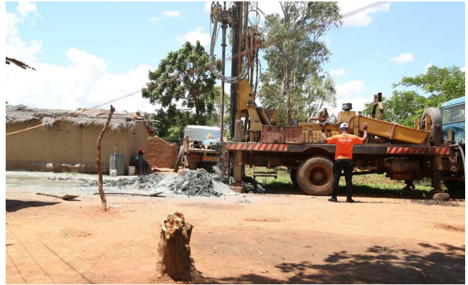
World Vision Malawi's drilling team is hard at work constructing a new site.
